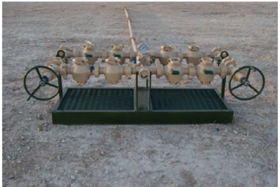
Plug Valve Manifold
